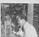
At work checking switches at Automatic Electric
